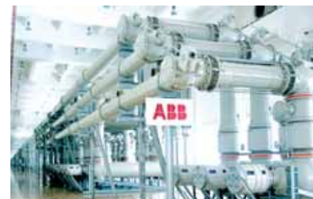
220 kV gas insulated substation
