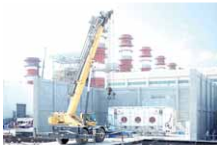
Field service and maintenance
