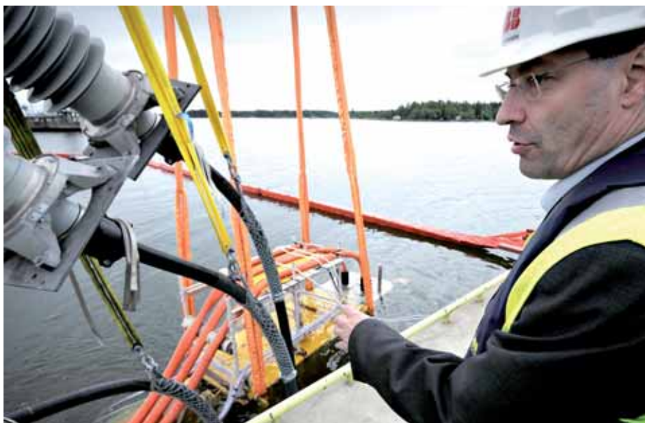
Testing of the subsea transformer
