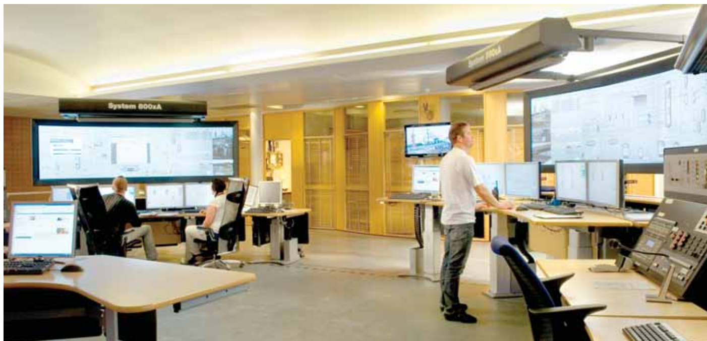
Control room using 800xA platform
