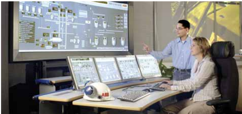
Control system operator workplace
