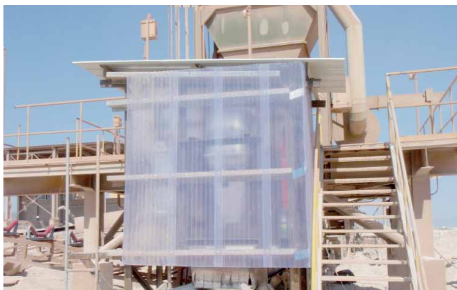
SpectraFlow™ in operation at Raysut Cement
