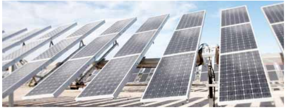
Panels at a solar power plant in Spain
