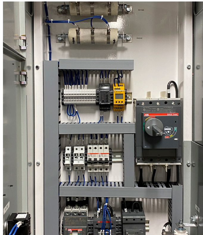
Custom built DC MCC panel
