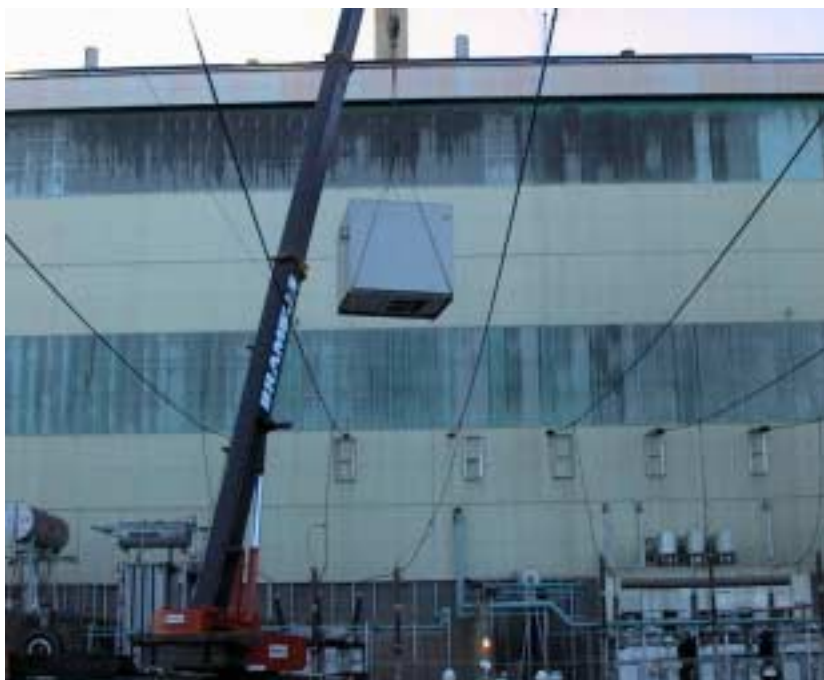
6.6 KV 2500 A 40kA Station Tie Switchboard / Switchroom being installed at NRG Gladstone Power Station.
