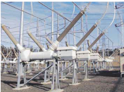
NCITs installed on Hybrid Breaker Bushing
