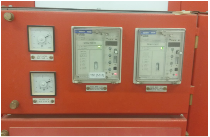
The existing SPACOM relays
