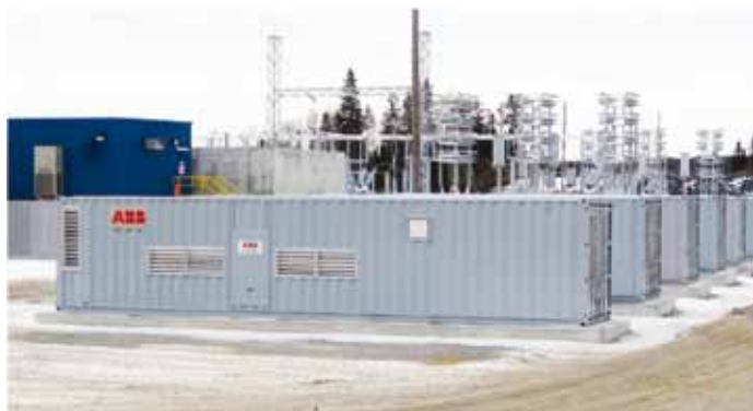
6 x 4.5 MVAR mining application for Canadian mine
