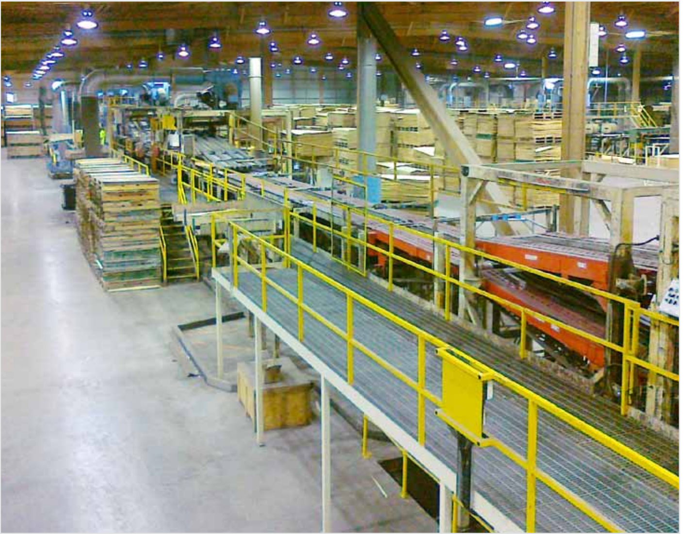
Carter Holt Harvey's Active Voltage Conditioner (AVC) protected production line
