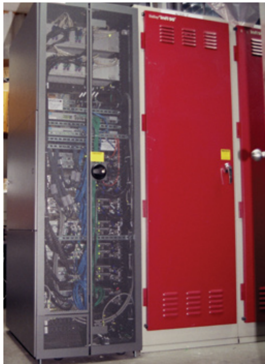
New System 800xA cabinet (left) next to INFI 90 cabinets (right).
