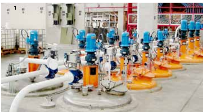
1 Letdown tanks fed by pigging lines | 2 Pneumatic transport system on top of powder silos
