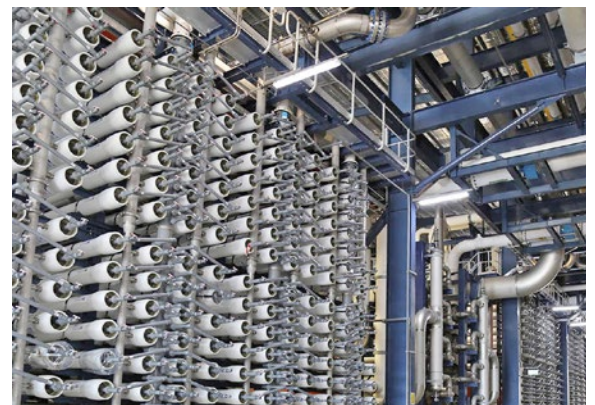
— The Gold Coast desalination plant uses a process called reverse osmosis, where pressurized intake water is forced through a semi-permeable membrane.
