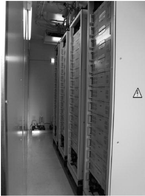
Fig. 6: Li-ion battery cubicles
