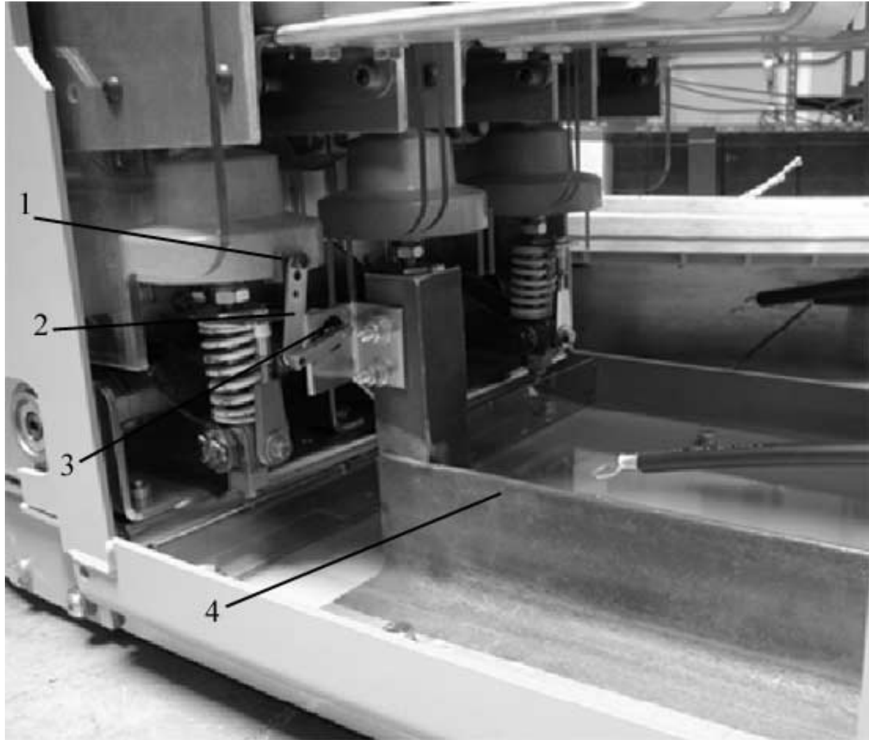
Figure 28. Travel Transducer Installation (Part # 0144D1238G001)
