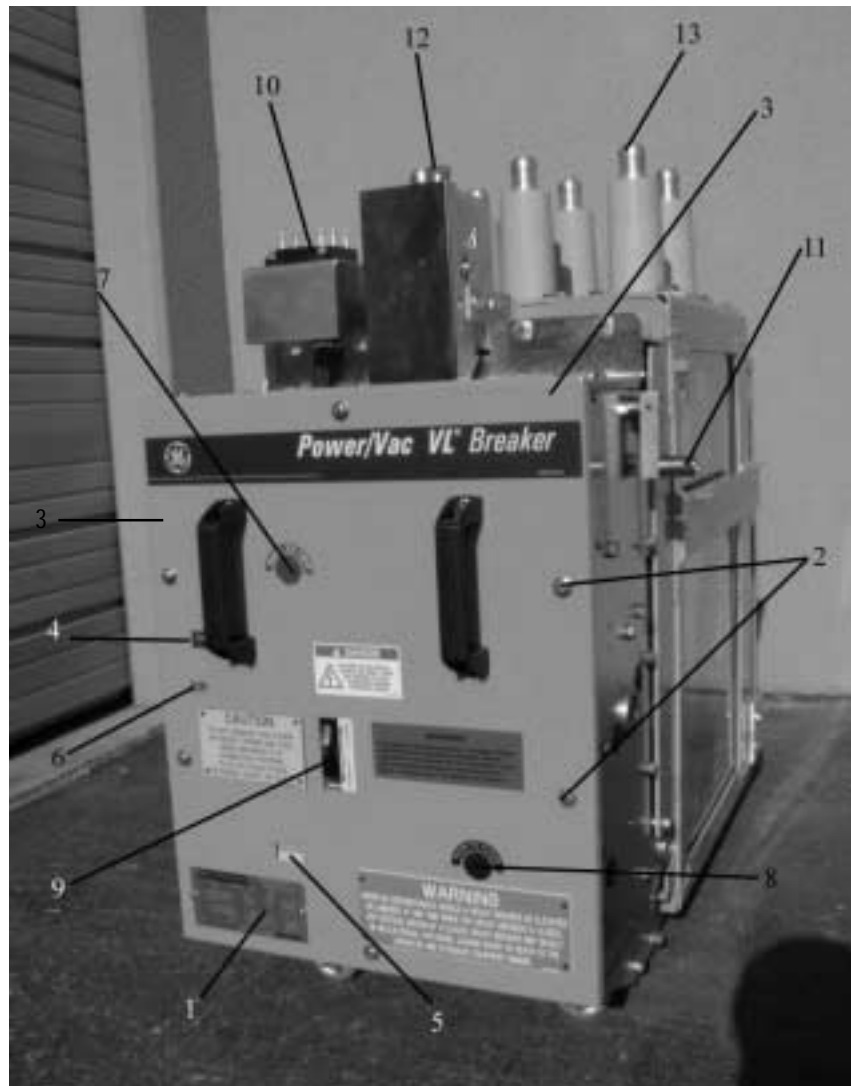
Figure 1. View of 5kV 'VL' Breaker with Front Cover
