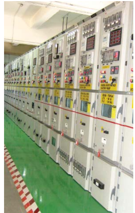
ABB installations at the plant
