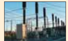
245 kV Spring Spring Breaker
