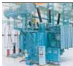
Power Transformer & Breakers
