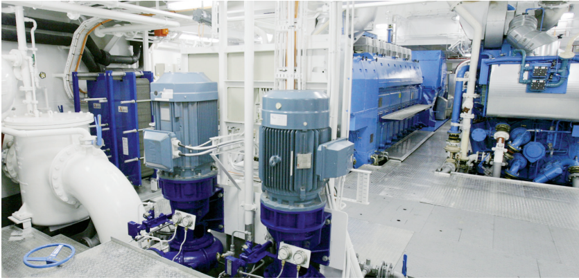
— Sea water cooling pumps with ABB high efficiency low voltage motors.
