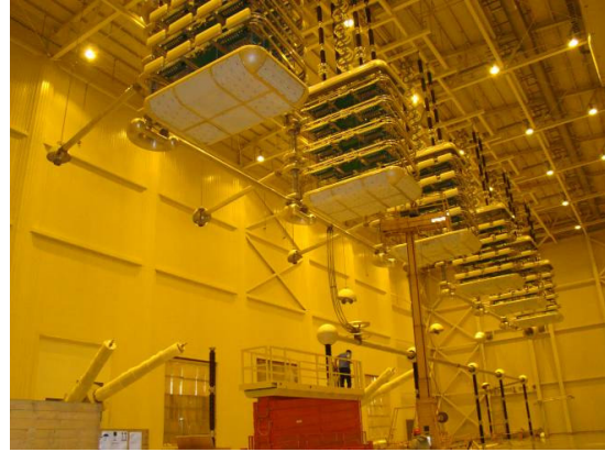
Figure 4. 800 kV dc valve hall
