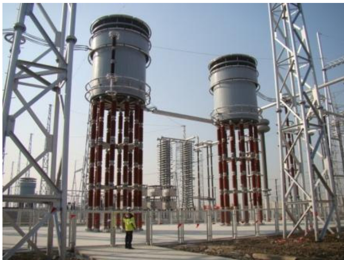
Figure 7. 800 kV dc smoothing reactors.
