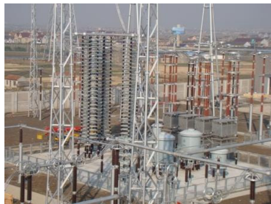
Figure 6. 800 kV dc filter
