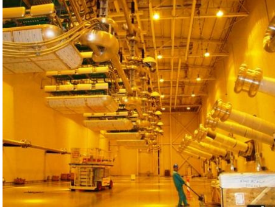
Figure 3. 400 kV dc valve hall
