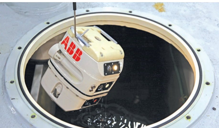
— 01 Insertion of the TXplore™ system through a transformer opening
