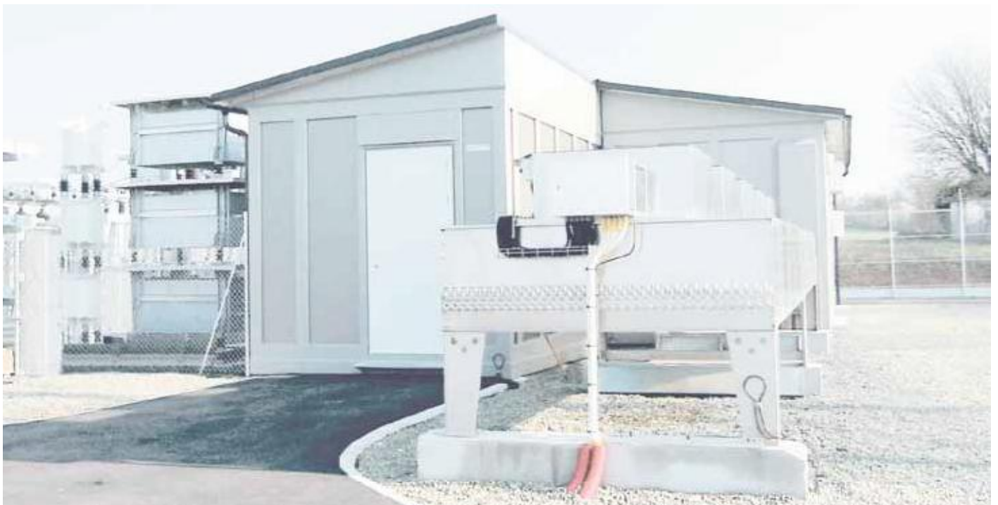
Fig. 1: SVC Light for railway load balancing
