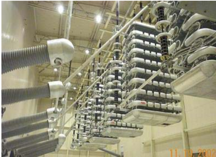
Converter valves in the Three Gorges-Changzhou transmission
