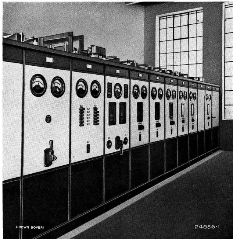
Fig. 13. — Sebrowitz Substation; front view of the direct-current switchboard.
