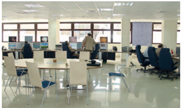
ECC's control room
