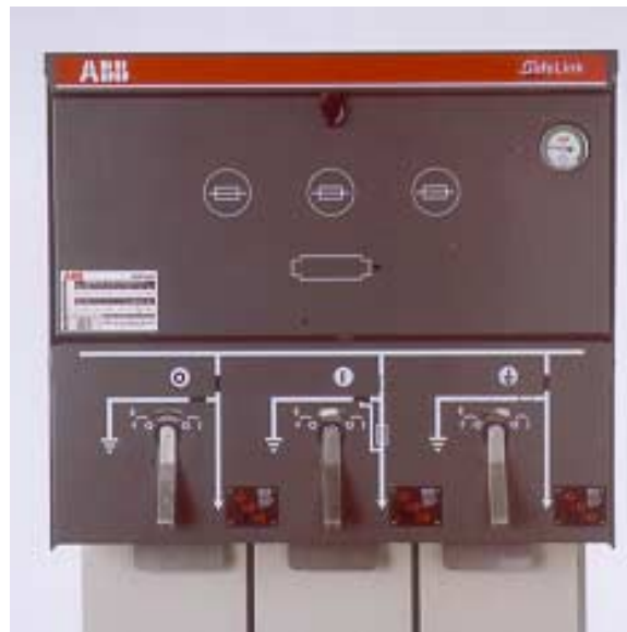
Figure 6: Front of SafeLink unit showing the mimic diagram and switches in (from left to right) the off, on, and earth positions.
