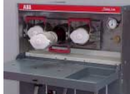
Figure 9: Central fuse assembly and fuse being withdrawn.
