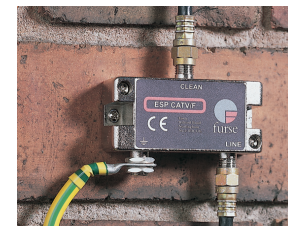
Figure 3. ESP CATV/F mounted in a garage near where the cable enters the building.
