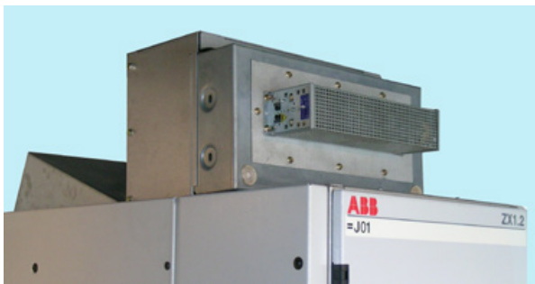
Fig. 7.8.5.1: Voltage transformers on a cable termination panel
