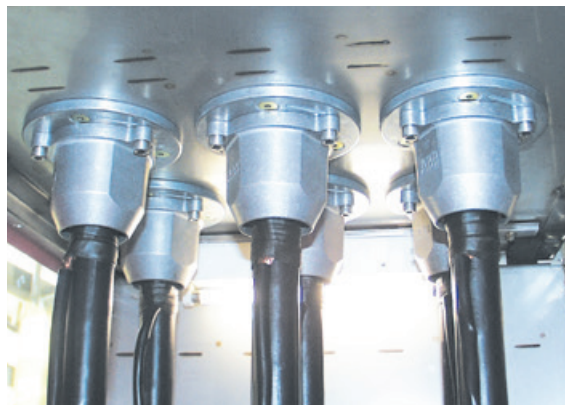
Fig. 7.4.1.1: View into the cable termination compartment in air with cable connectors and cables
