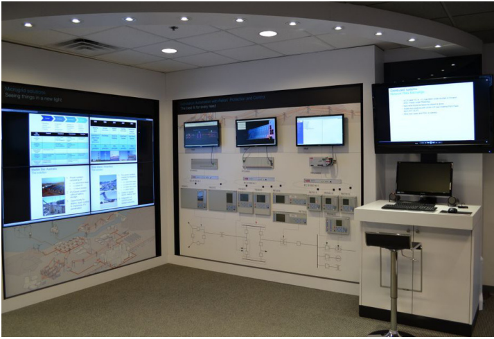
Microgrid, MicroSCADA, and Relion® wall
