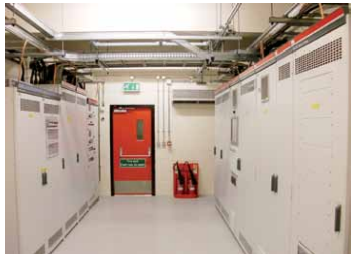
Fig. 5: MACH 2 control system (right) and relay protection cubicles (left)
