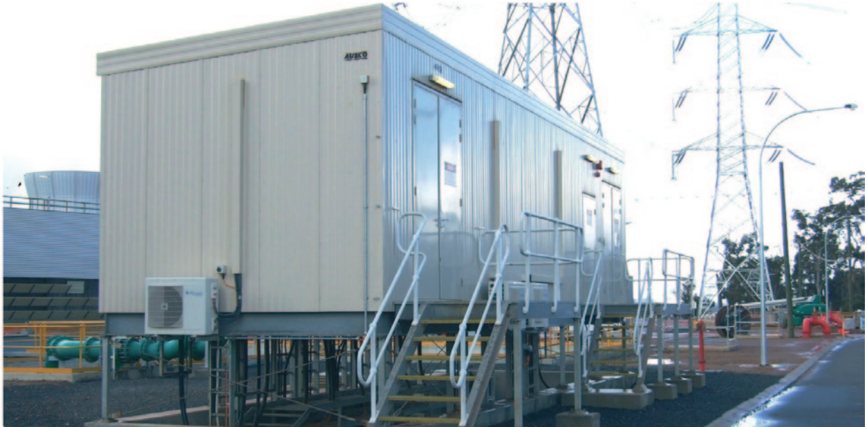
Typical E-House Installation
