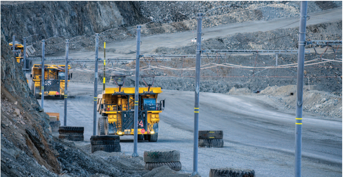
In a studied section, haul trucks connected to the trolley assist system reduced their carbon dioxide equivalent per truck cycle by 79 kilograms.
