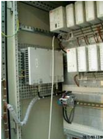
PLC AC80 with I/O S800
