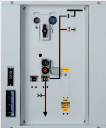
Controls for switching devices
