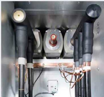
Cable compartment with current transformers
