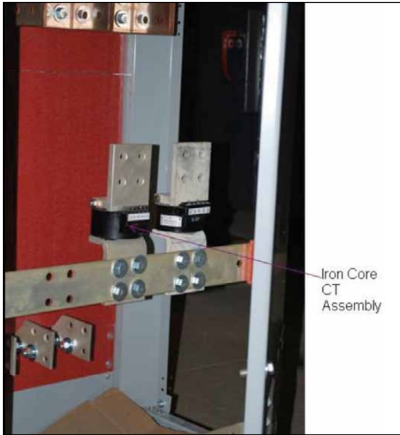
Figure 1. Neutral—AK25/50 Iron Core Current Transformer Assembly
