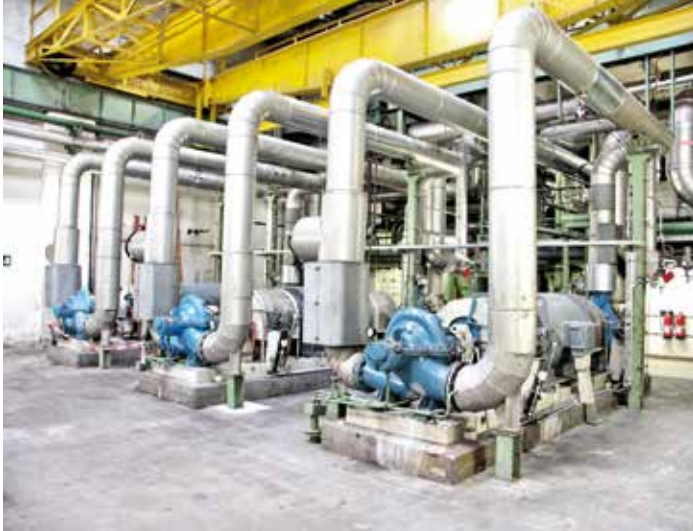
1 District heating pumps | 2 Control hierarchy
