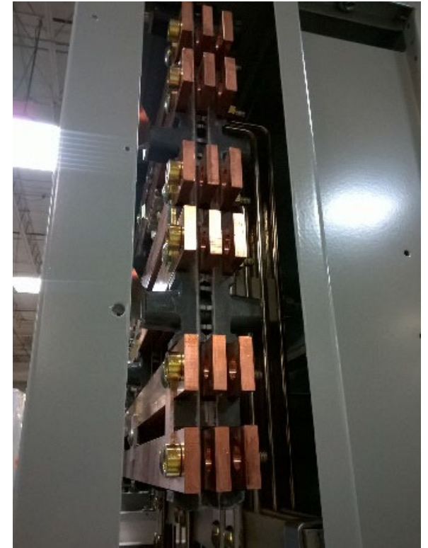
1.5" main bus (side view)
