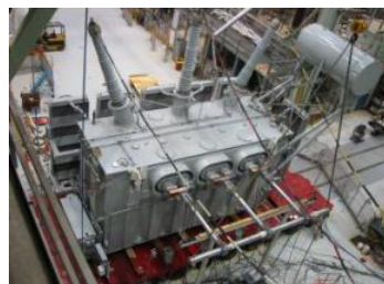
Figure 3: Transformer during factory tests
