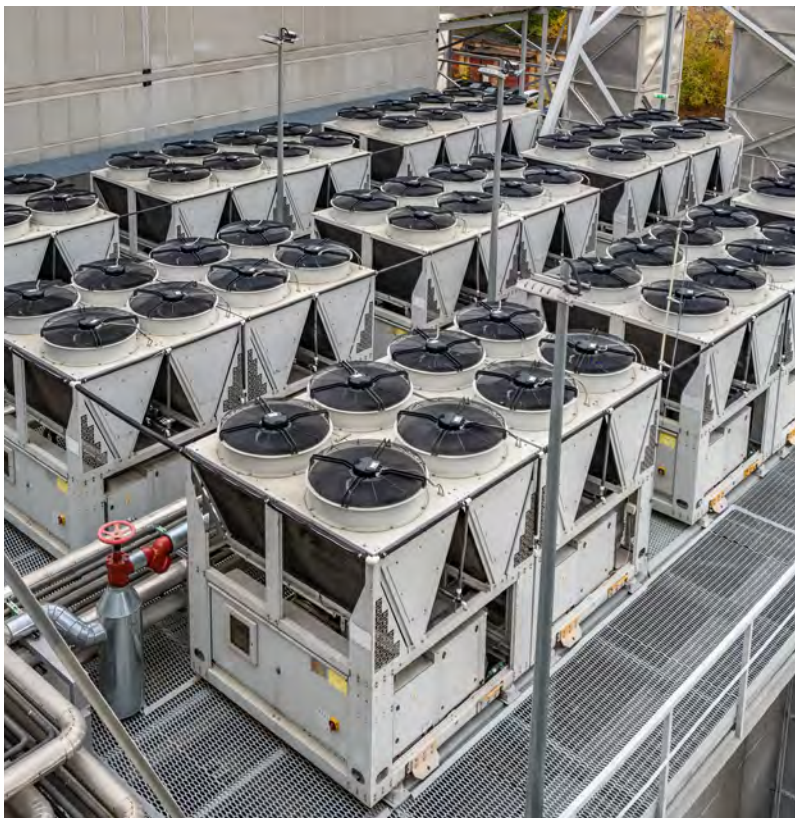
Air-cooled chillers on a rooftop of a data center. Photo source: Adobe stock image
