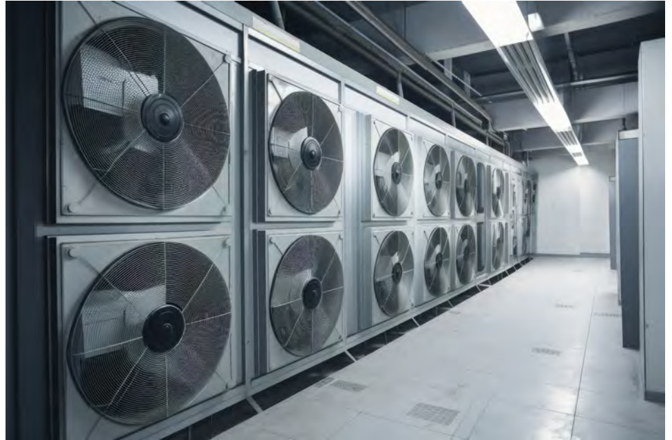
A fan wall in a data center. Photo source: Adobe stock image
