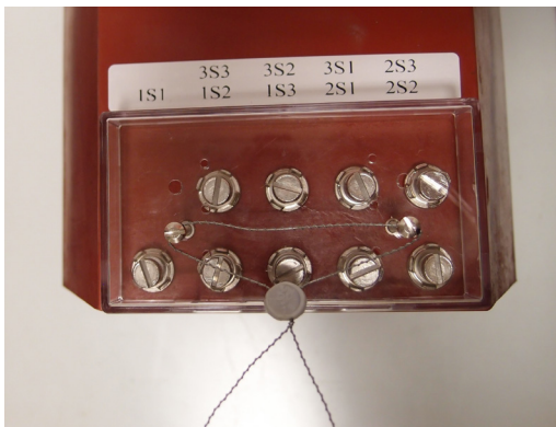
08 Sealing of secondary terminals for tariff metering
