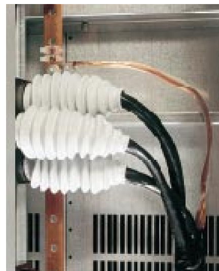
The cable compartment of the apparatus cubicles has ample space for the connection of outgoing cables.
