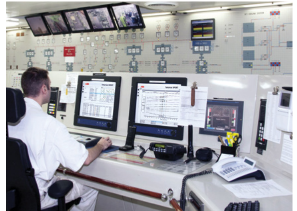
— Tekomar XPERT control room
