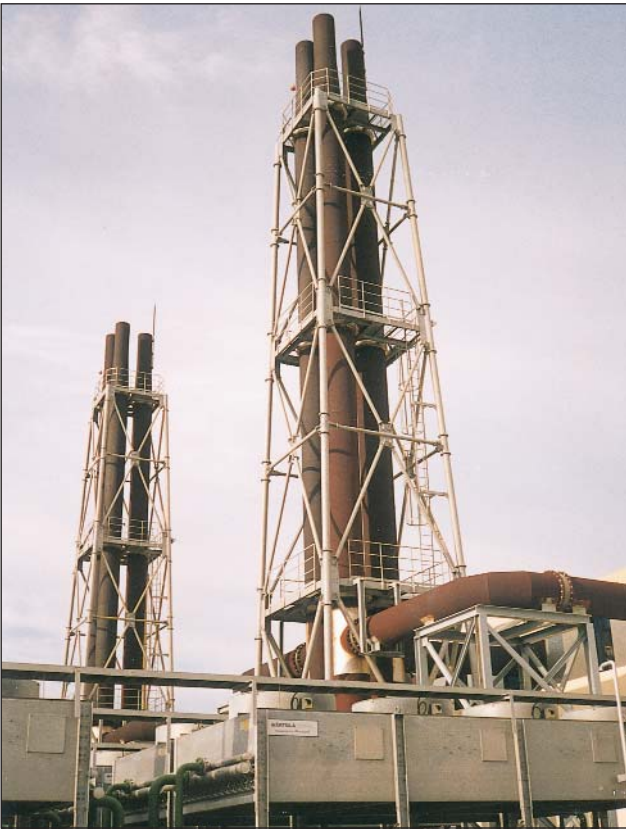
Part of the power plant.
