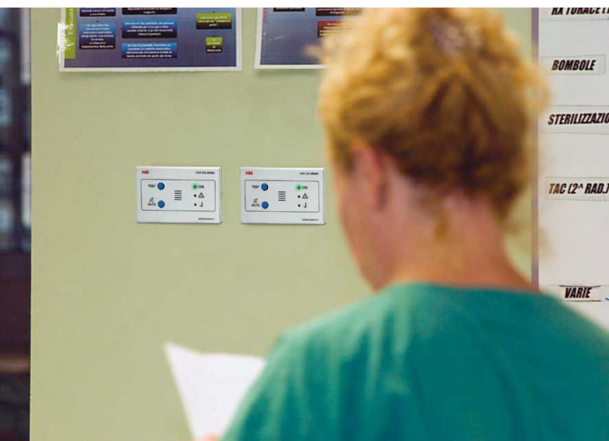
Figure 3.8: QSD remote signalling panels allow medical personnel to be immediately aware of malfunction situations
