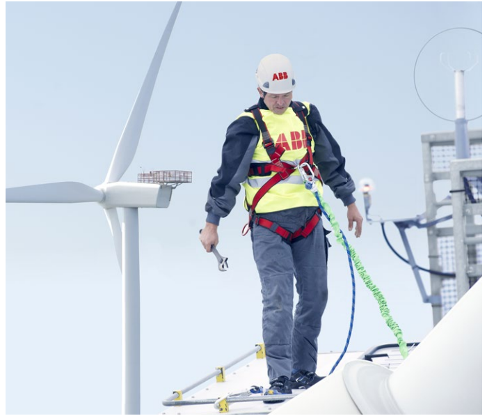
ABB field service engineer during commissioning
