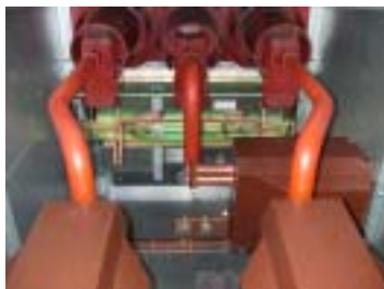
Feeder compartment : Lower bushings, current transformers and branch connectors.
