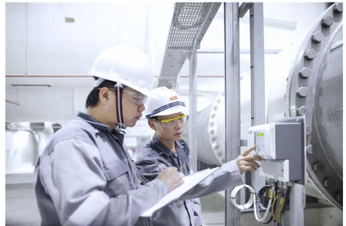
Photo: ABB ProcessMaster electromagnetic flowmeter being serviced
