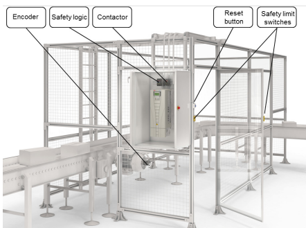
Figure. 7. Safety monitors receiving and sending safety impulses to the drive. More safety devices and wiring are needed compared to integrated drive-based functional safety (see fig. 8)
