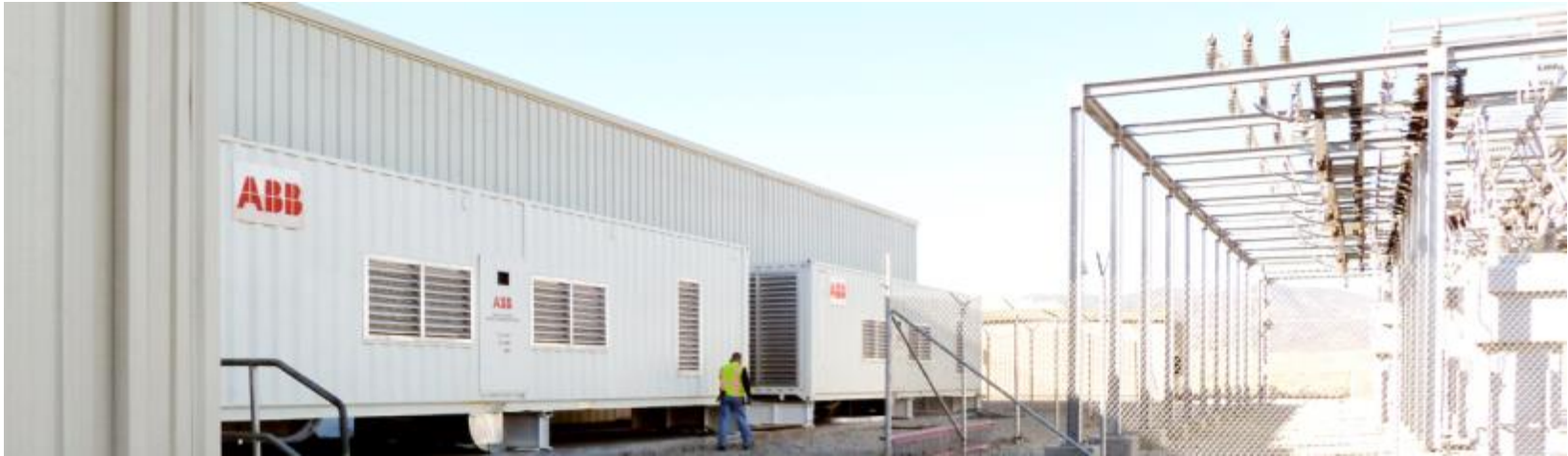
8 MW / 32 MWhr Tehachapi Storage Project
