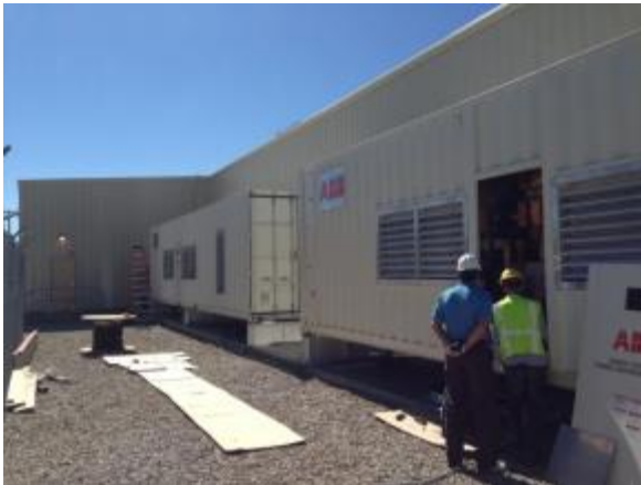
8 MW / 32 MWhr Tehachapi Storage Project
