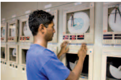
The process lines at Sappi Saiccor have been controlled by ABB's automation systems since 1994.
