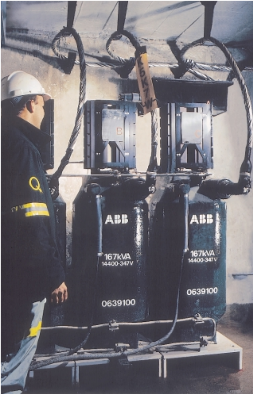
First series of Solid Insulation Distribution Transformers installed in a Hydro-Québec underground vault
