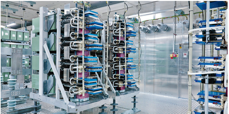
Figure 3: Modular H-bridge units, 2 stacks of 4 modules each
