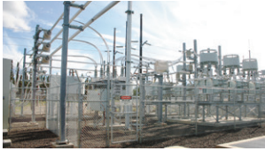
SVC for pipeline drive.
