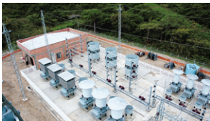
SVC supporting the feeder voltage of an oil field.
