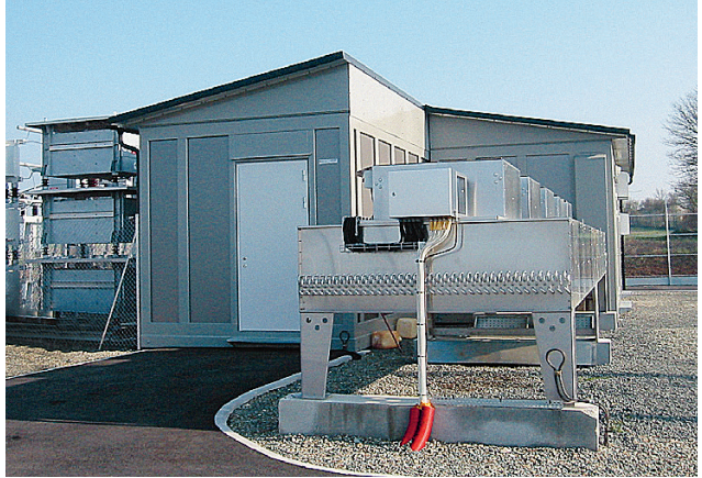
A site view of the Load balancer
