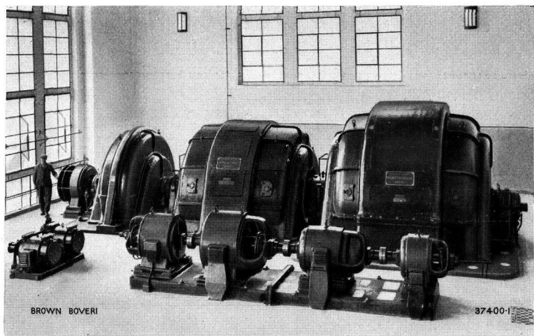
Fig. 10. — Converter set and auxiliaries in machine-hall of Mühleberg Power Station.
