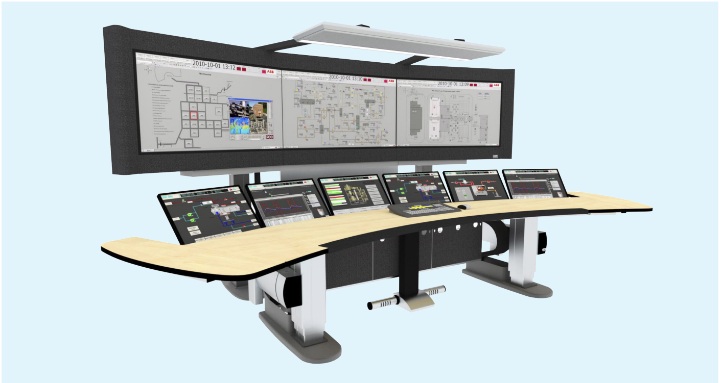
A System 800xA EOW-x extended operator workstation similar to this provides operators at AkzoNobel in Örnsköldsvik, Sweden, with better overviews and clearer process information.
