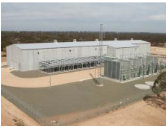
Converter station at Berri.
